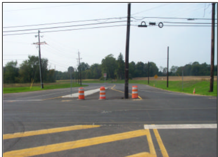
Utility relocation delay can have cost and safety implications
